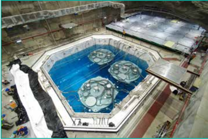
The Far Hall (EH3) water pool with 3 Anti-neutrino detectors in place before the pool cover is installed.
