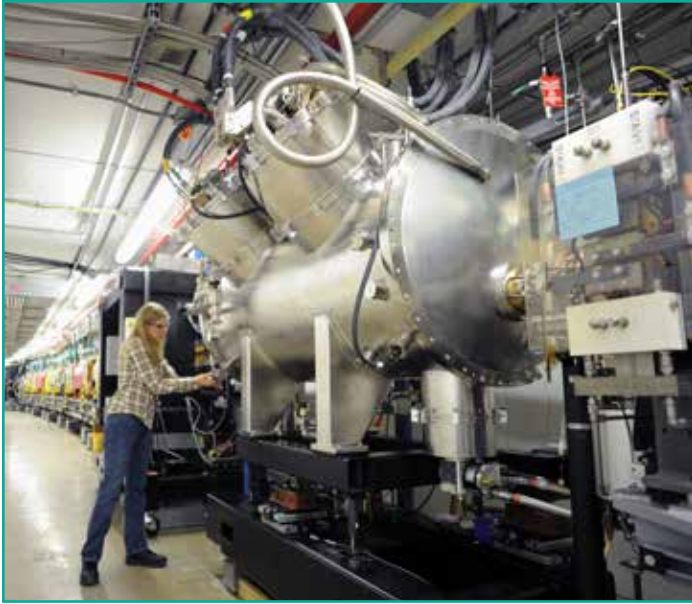
APS – Upgrade of superconducting ID
